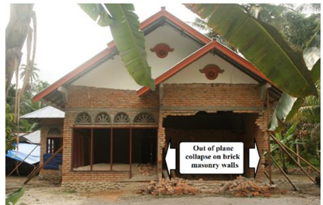
(b) Absence of RC tie-beams and tie-columns
