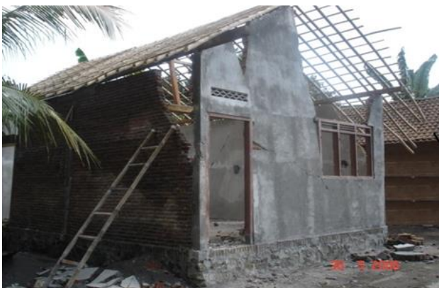
(a) Incorrect prevailing practice of RC frame
