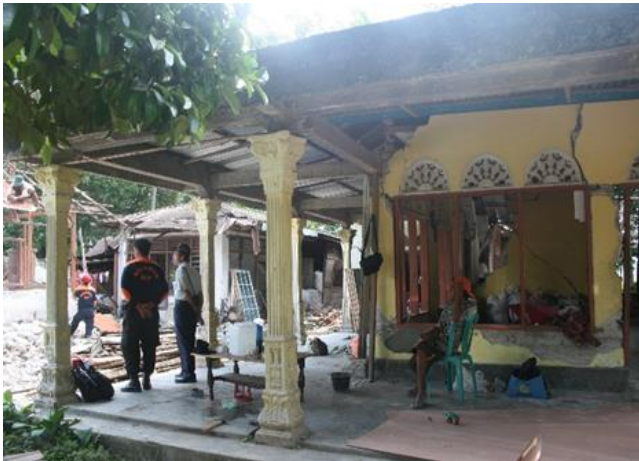
(a) Improper RC additional canopy (Padang Pariaman)
