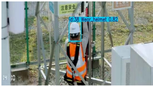
(a) Workers' accidental entry into hazardous areas
