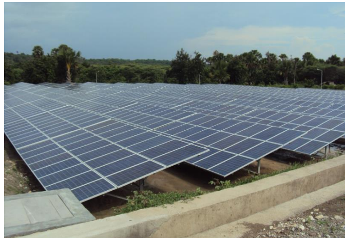
Fig. 3 Photo of array Kupang PV plant
