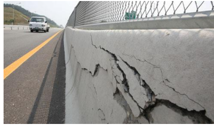
Fig. 2 Crack in barrier
